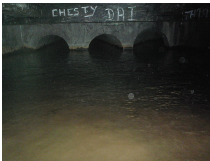
Inside the chamber – silt to half depth of pipework
